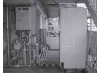
Group of domestic hot water systems placed in the hallway of multi-family type test building
