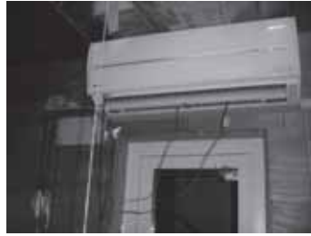
Measuring of air conditioner load efficiency
