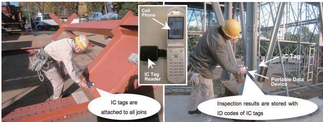
Photo 3. Left, inspecting the members of a building framework; right, inspecting the condition of bolted joints of a steel structure. Both of these inspections use IC tags. The IC tags are used to display information required for various inspections on portable devices. Center, cell phone with an IC tag reader attached.
