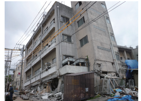
Photo 7: Floor collapse on the first floor of a piloti structure
