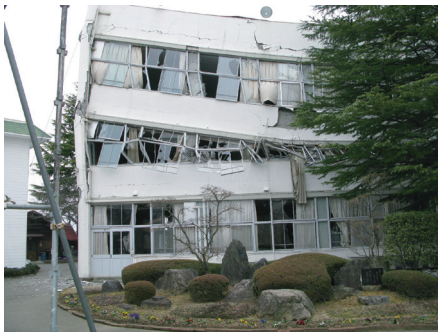
Photo 1: Mid-story collapse in a low-rise building
