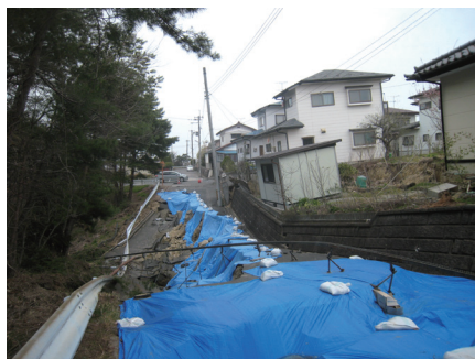
Photo 11: Damage due to a landslide from a sloped edge
