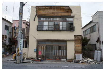
Photo 2: Fallen parts of exterior walls
