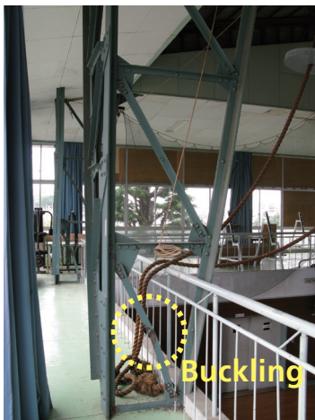
Photo 6: Buckling of diagonal bracing of lattice columns (part shown with yellow dotted line)
