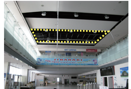
Photo 13: Fallen ceiling at an airport departure lobby (yellow dotted line indicates where the ceiling droppage occurred)
