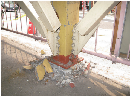
Photo 4: Damage to exposed column bases
