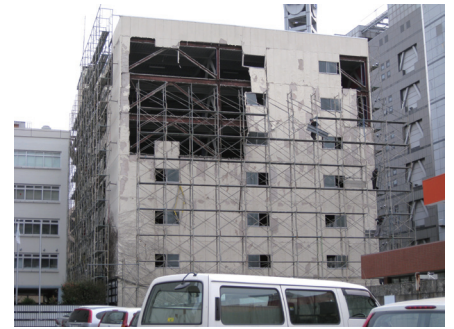
Photo 12: Fallen exterior wall panels
