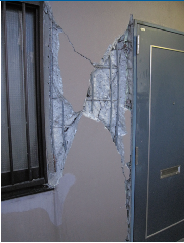
Photo 9: Non-structural shear failure
