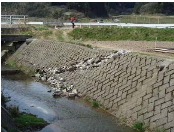
F-c 護岸の破壊状況 2
