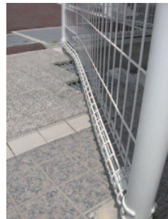
(c) 侵入防止柵のゆがみ
