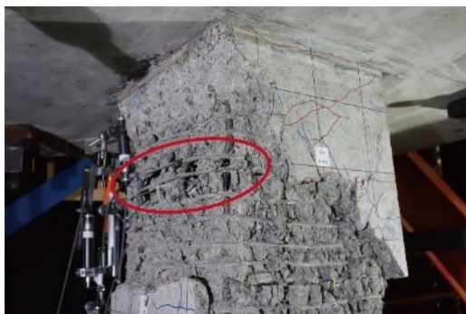
(c)北面柱頭主筋の座屈
